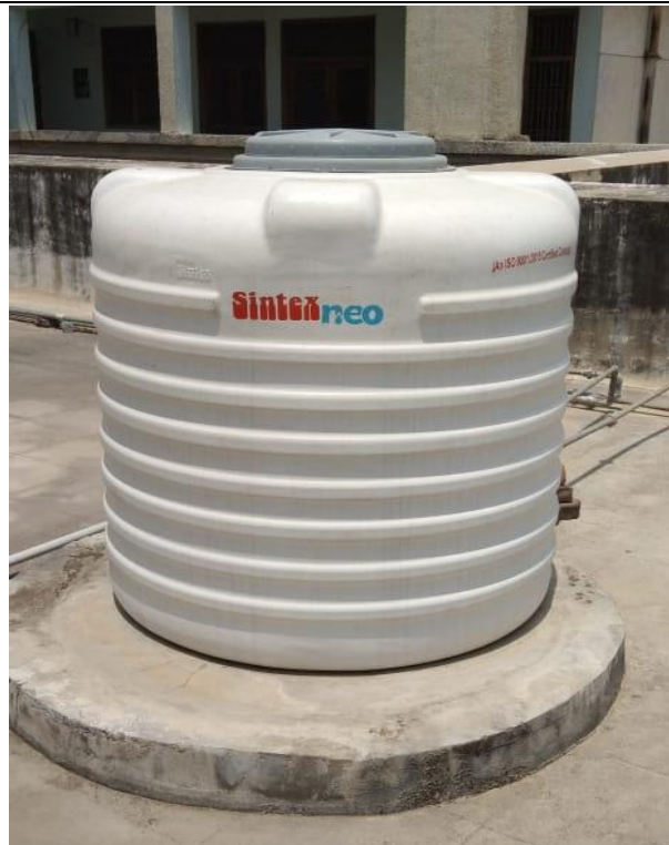
RO Treated water storage tanks
